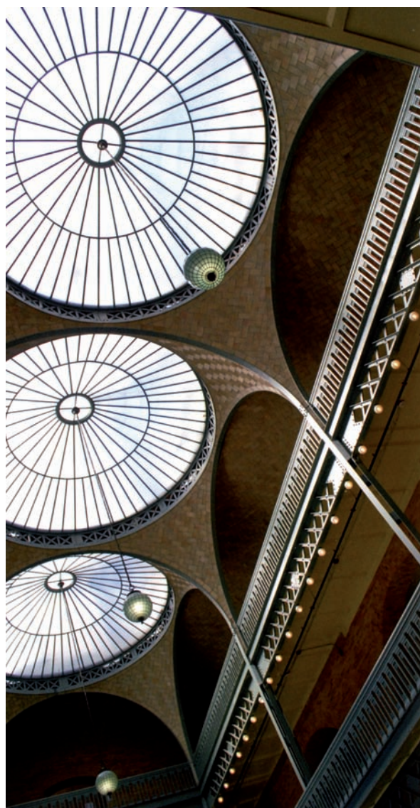
Guastavino Co. con John Galen Howard, Hearst Memorial Mining Building, ahora Department of Material Science and Mineral Engineering, University of California, 1902, Berkeley.
